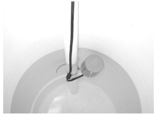
High Water; Switch Off
